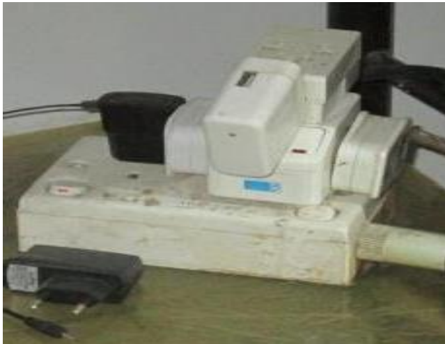
Overloaded electrical power point
