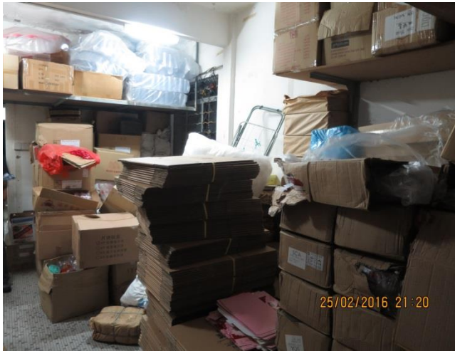
Fire hazard materials and obstruction of exit
