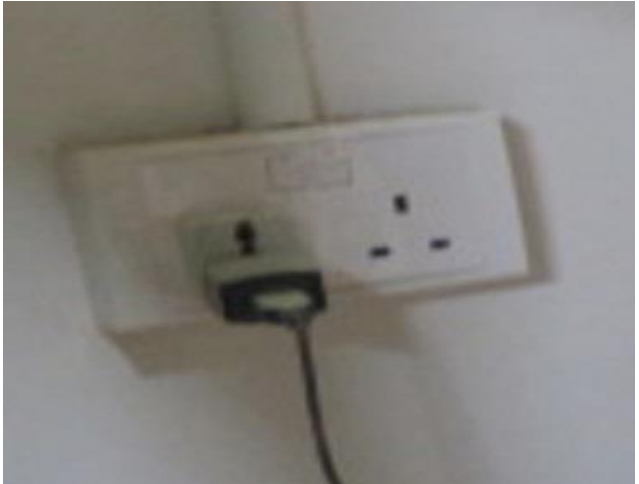
Correct use of power point
