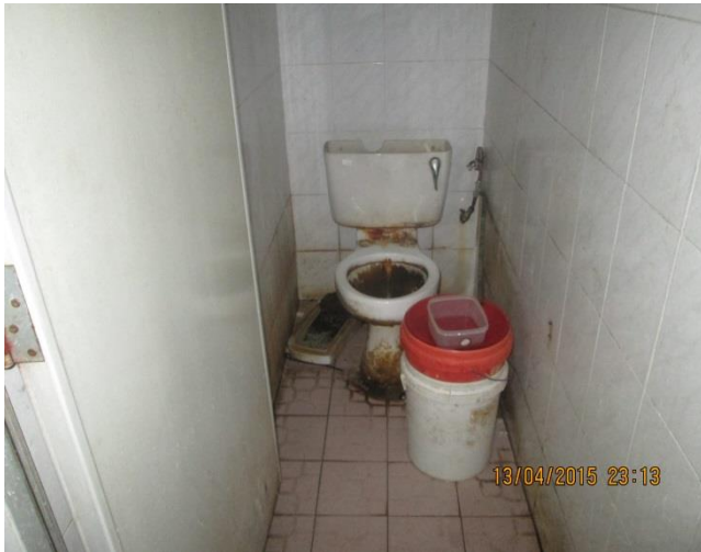
Poorly maintained sanitary facilities
