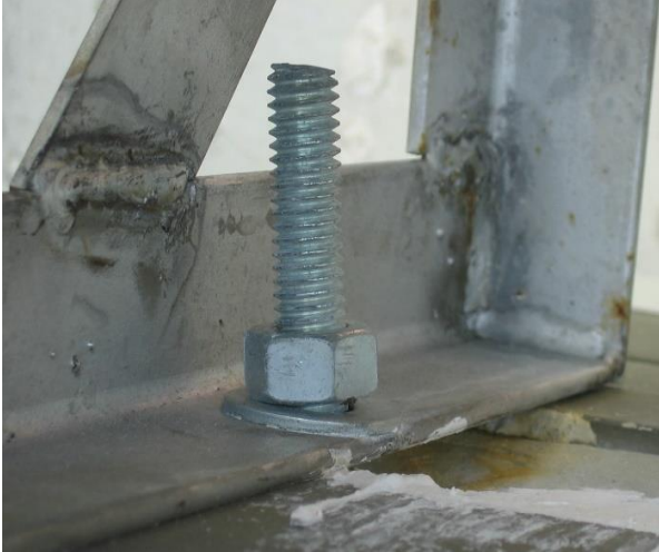
Figure 3: Loosened bolt and nut
